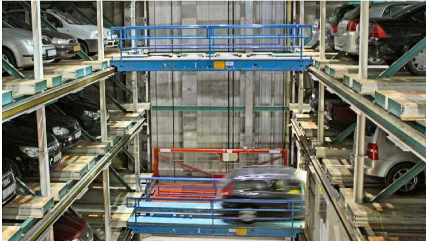
Figure 48 Automated Parking Facility (top) and Mechanical Parking Lift (bottom)
