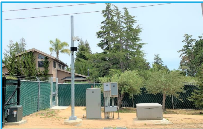
Photo 22: GHWTP Entrance Improvements - New Electrical Cabinets, Conduit, and Pull Boxes Located next to the New Entry Gates on the Inside
