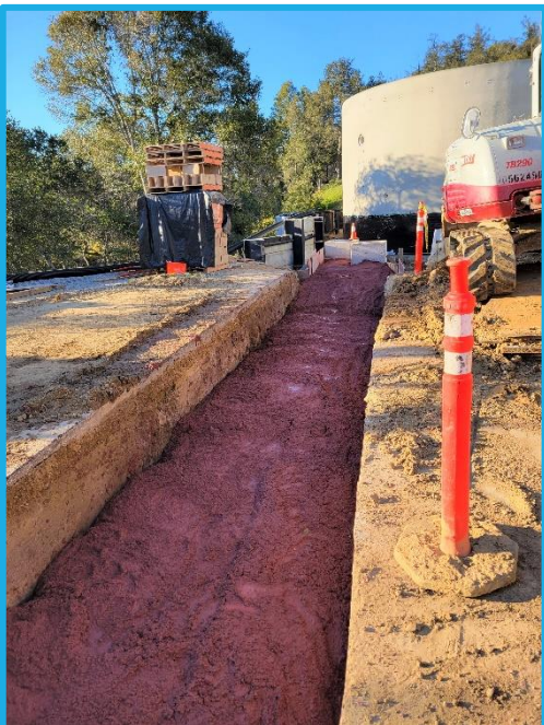
Photo 16: GHWTP Concrete Tanks Replacement – Pouring Red Concrete on the Electrical Ductbank near the New Concrete Tanks
