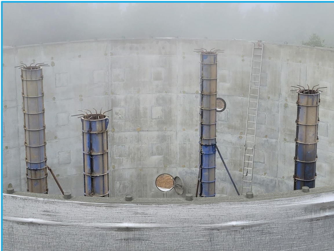
Photo 13: Graham Hill WTP Concrete Tanks Replacement – Installed Rebar and Column Metal Forms at the Reclaim Tank
