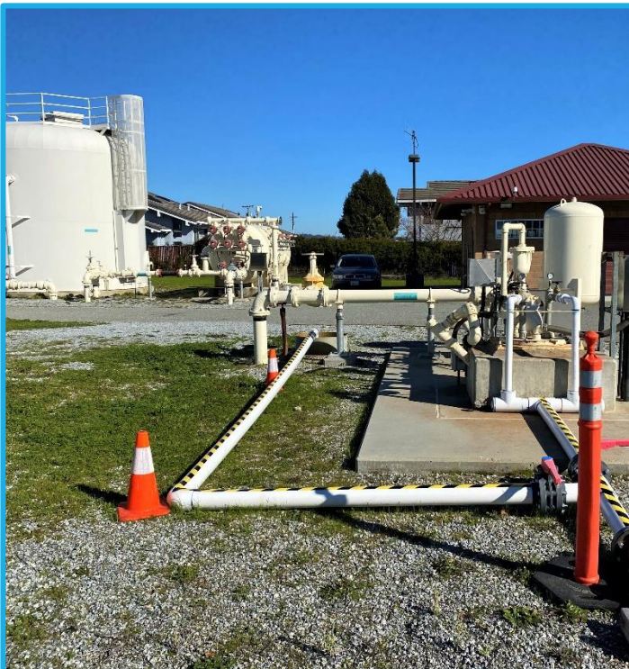
Photo 3: Beltz 12 Well - Injection Drop Tubes and Temporary Piping Setup at Beltz 12 for ASR Demonstration Study Year 2
