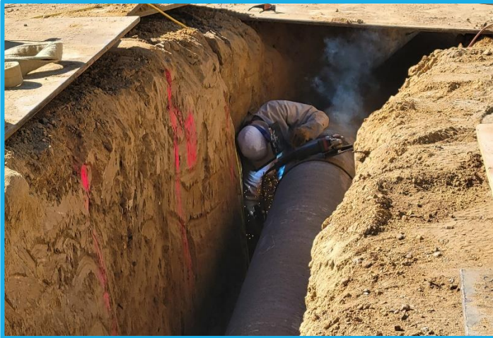
Photo 14: GHWTP Concrete Tanks Replacement - Contractor's Certified Welder Welding the 16-inch Treated Water Steel Piping on the Access Road
