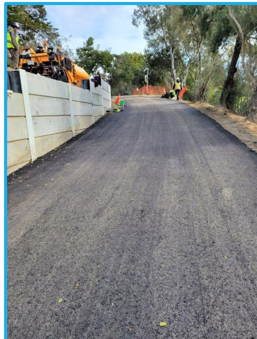
Photo 17: GHWTP Concrete Tanks Replacement – Installed Overlay of 2 1/2-inch Asphalt on the Access Road
