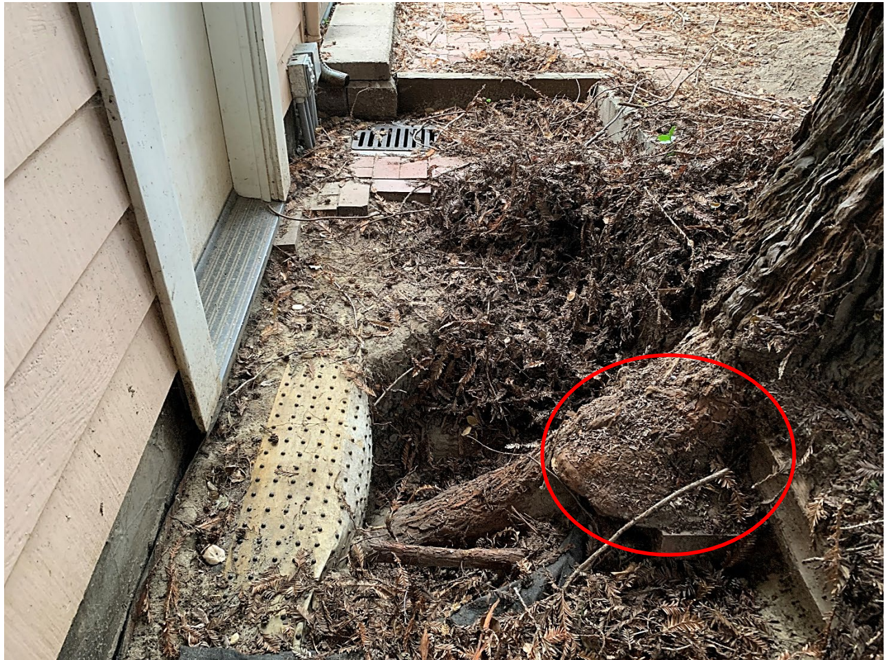
Image #7 –Tree T2, view of root and trunk buttress. (circled), growing towards foundation and doorway.
