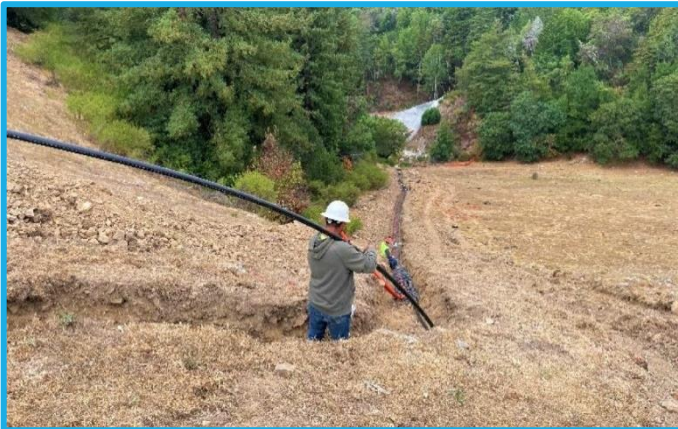
Photo 7: Newell Creek Dam Inlet/Outlet Replacement – Installation of Electrical for Dam Face Ductbank
