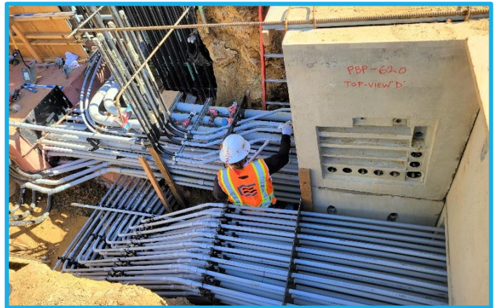
Photo 12: GHWTP Concrete Tanks Replacement – Installing Conduit in Ductbank between the New Electrical Building and Electrical Vaults
